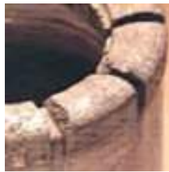
LOSS OF INSIDE DIAMETER
